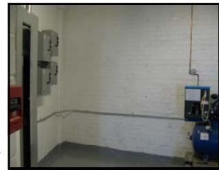
Mechanical Room June 19, 2009
