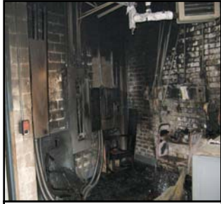
Mechanical Room July 25, 2008
